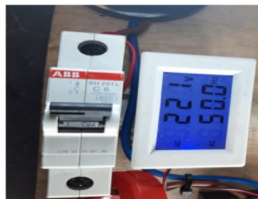
Figure 6. MCB AC With Voltage And Current Meters
