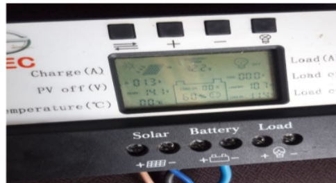
Figure 5. Solar Charge Controlled (SCC)
