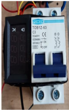
Fig. 7. DC MCB With Voltmeter And Amperemeters
