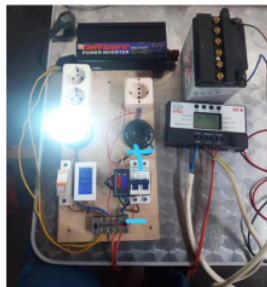
Fig. 8. Test circuit using DC MCB and AC MCB with Voltampere and Amperemeters
