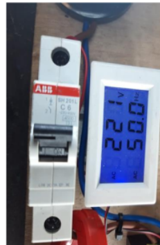
Fig. 6. AC MCB With Voltage And Current Meters
