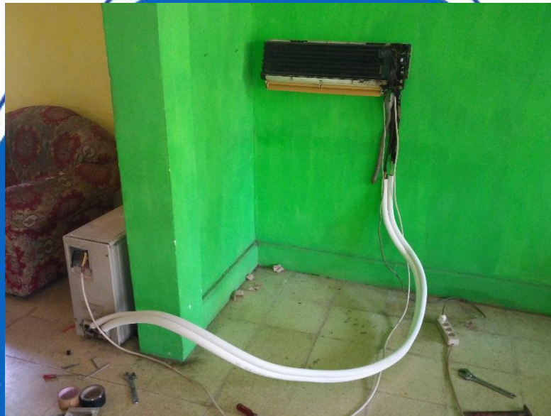
Gambar 4.3. Unit Indoor dan Outdoor Air Condition (AC)
