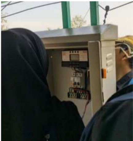
Figure 3. Panel Box Outside
