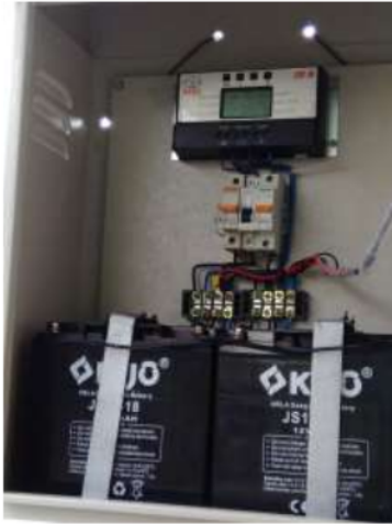
Figure 2. Inside Panel Box
