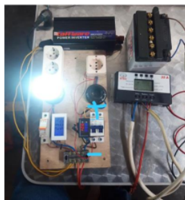
Fig. 8. Test circuit using DC MCB and AC MCB with Voltampere and Amperemeters
